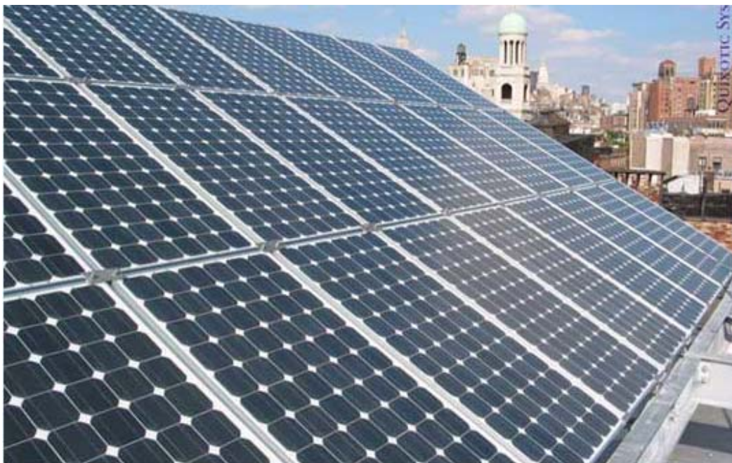
A rooftop PV installation
