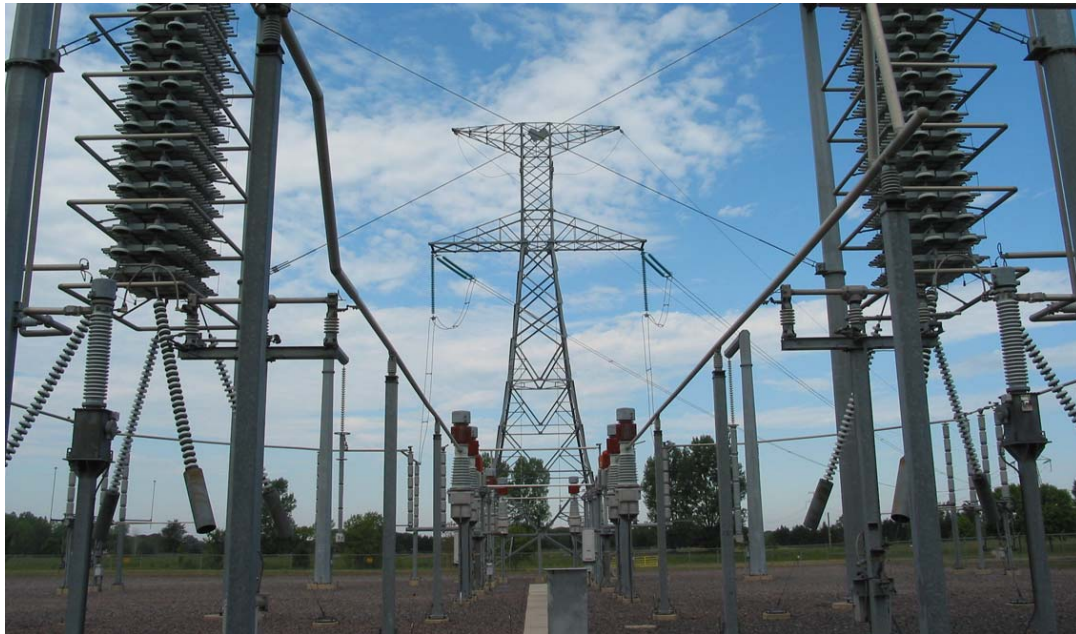
DC Line at the Dickinson HVDC Converter Station, Minnesota
